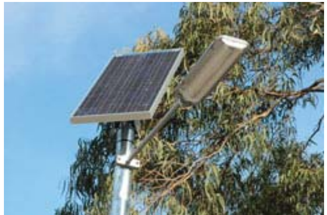
Solar street lights at Brickpitt Park, Thornleigh
