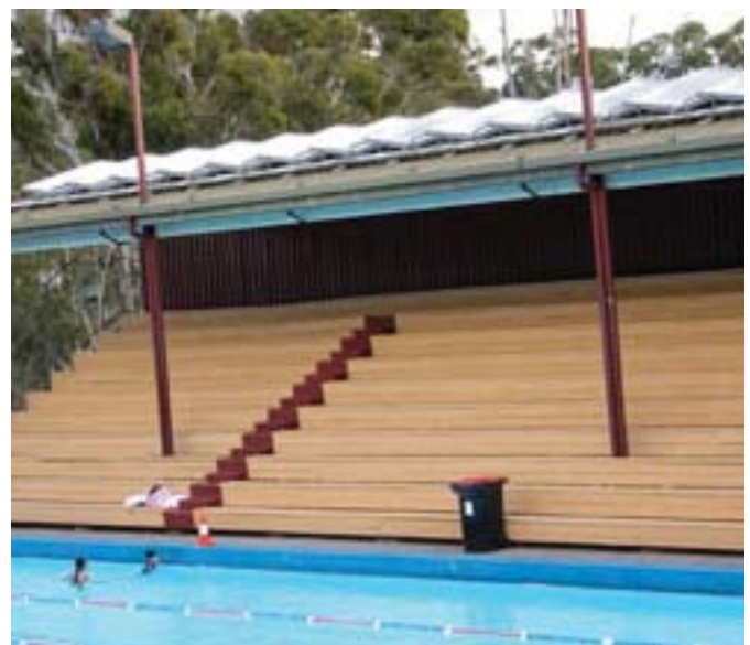
Solar collectors at Hornsby Aquatic Centre
