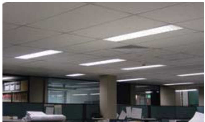
Energy efficient office lighting and controls
