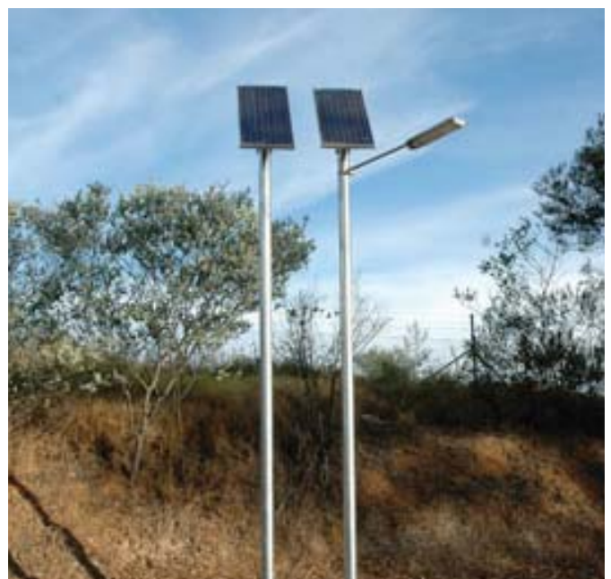
Solar street lights at Brickpitt Park, Thornleigh
